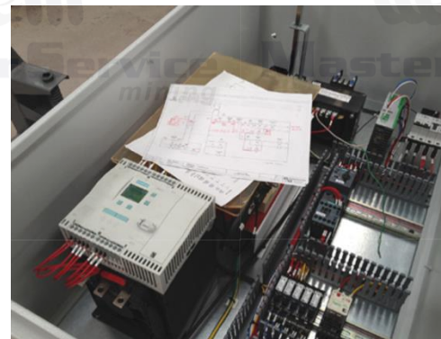
Gabinete Soft Starter y PLC
